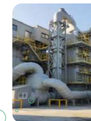
TS-3 SCR denitrification equipment
