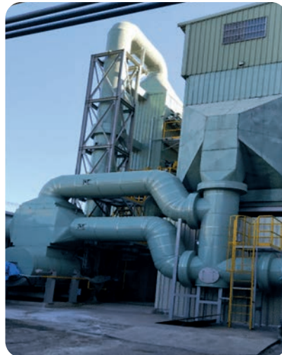
TS-7 SCR denitration equipment
