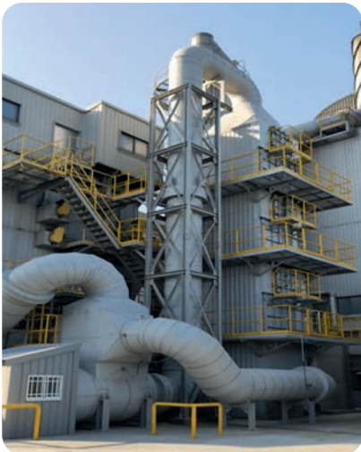
TS-3 SCR denitration equipment
